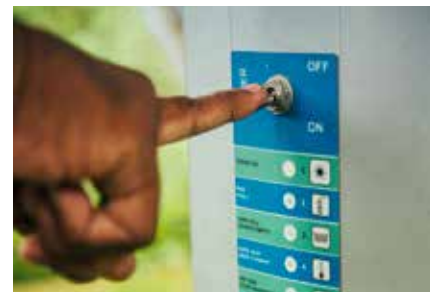
The solar-powered wells will replace, on an annual basis, 110 million tons of CO 2 emissions from AC pumps and 20 million tons from diesel pumps.
